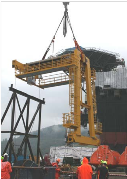
At the Westcon yard the bridge, A-frame and track beam have been assembled before the crane system was transported to its final site on the rig.
